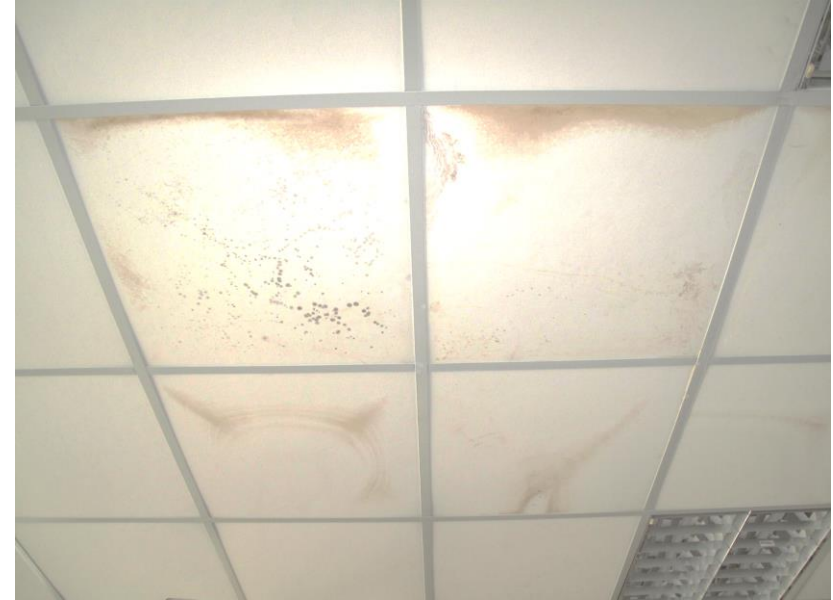
Mold/fungus on ceiling
