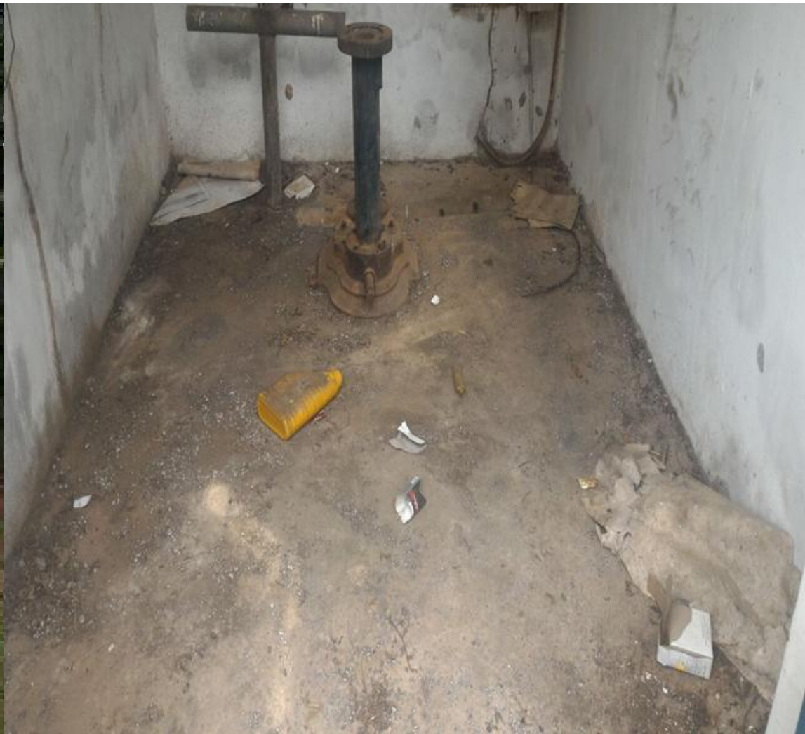
Mercury found scattered on the floor
