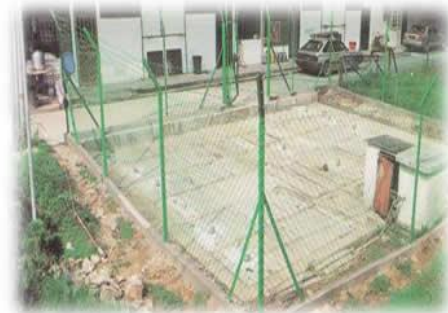
Communal Septic Tanks(CST)
